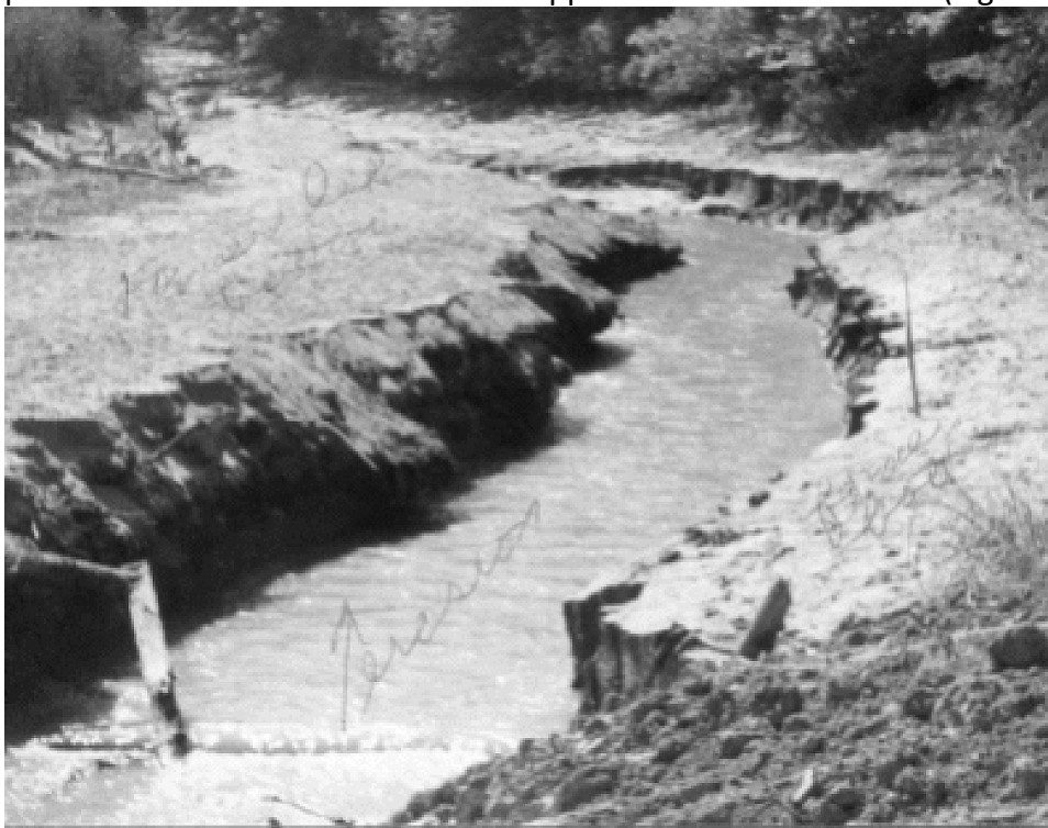
Figure 15. The channel just upstream from the dam on 3/27/1985 shortly after removal of the dam. View is from approximately same position as Fig. 14. PA DEP photo.
