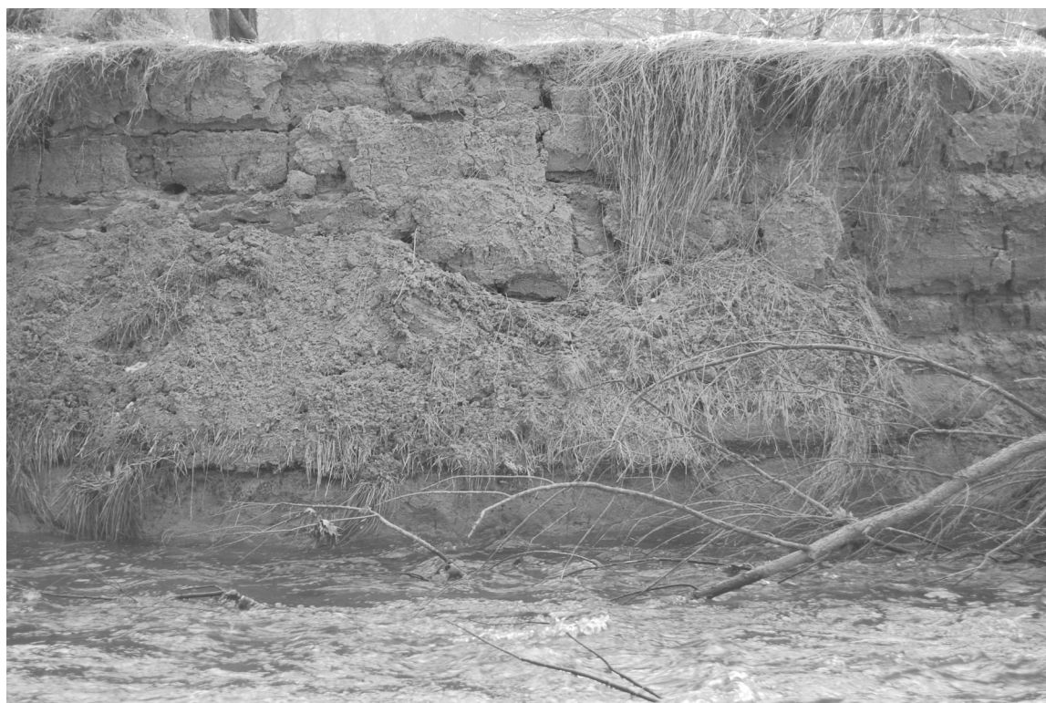
Figure 23. The bank below STOP D on 2/3/08. Note fractures in cohesive sediment, and accumulation of silty "crumbs" on bank from just above water to about half way up.
