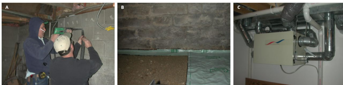
Figure 8. Stray CO 2 remediation, Geiwitz residence basement. A. Concrete foundations blocks were filled with a special grout mix to decrease permeability of the basement to gas. B. Vapor barriers installed to make subfloor impermeable to migrating gas. C. Vents were installed as was a fan system designed to create positive pressure beneath the home that maintains a meter-scale buffer zone between migrating CO 2 and the basement.
