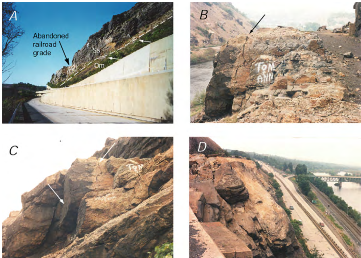
Figure 25. Rockfall hazard due to cross fractures along PA 248 and abandoned railroad grade in Lehigh Gap. A - Northbound lane of the highway, as it appeared in 2000, is cantilevered above the southbound lane beneath the contact between the Shawangunk Formation (Ss) and Martinsburg Formation (Om). The location of the highway was constrained by a railroad along the Lehigh River to the left and a railroad, now abandoned, above. A wire-meshed gabion (arrows) lines the edge of the railroad grade to protect against falling rocks; B - Cross joints in the Shawangunk Formation (arrow) opening parallel to the abandoned railroad grade, Lehigh River below; C - View of cross joints from highway below. Some of the rock has been removed subsequent to taking this picture in 1990; D - Cross joints in the Shawangunk Formation parallel the highway below.
