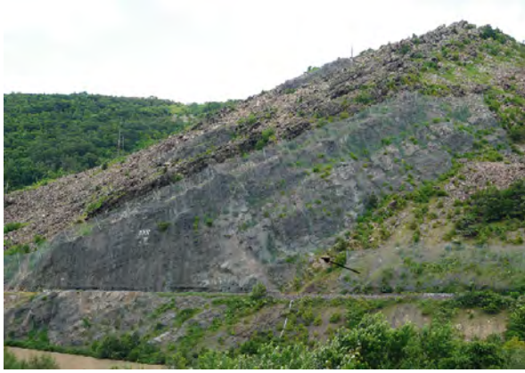
Figure 22. Wire mesh drapes cover much of the south slope of Blue Mountain in Lehigh Gap. Arrows points to Ordovician-Silurian contact. View taken across the Lehigh River from the Lehigh Gap Nature Center.
