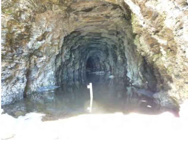
Figure 8. Close-up of the southeast portal of the O&W tunnel's east portal showing gently west-dipping bedding, water in tunnel (a constant problem during railroad operations), and lack of lining at portal.
