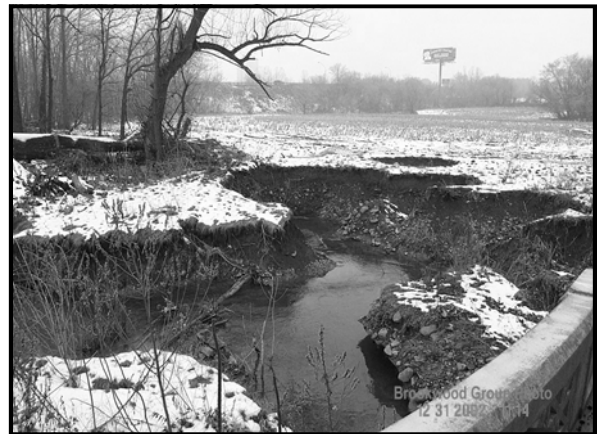
Figure 5. Coalescing sinkholes along the SR 107 bridge in 2002. Photo courtesy of the Brookwood Group.
