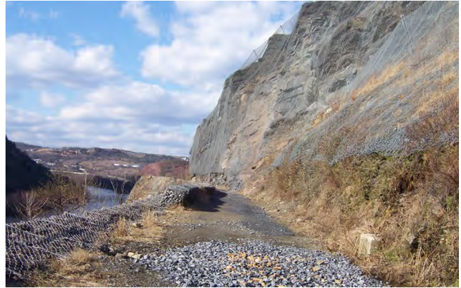
Figure 23. Much of the Shawangunk is covered in wire mesh drapes. Part of the Martinsburg in the foreground is also covered to prevent shale-chip spalling onto the roadbed.
