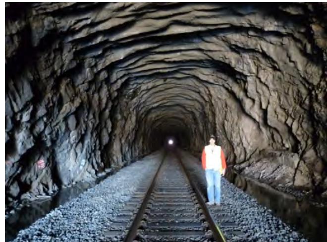
Figure 21. Unlined west part of the Erie Railroad tunnel at Otisville. The Shawangunk conglomerate here forms a ragged, but solid, arch that does not require lining.
