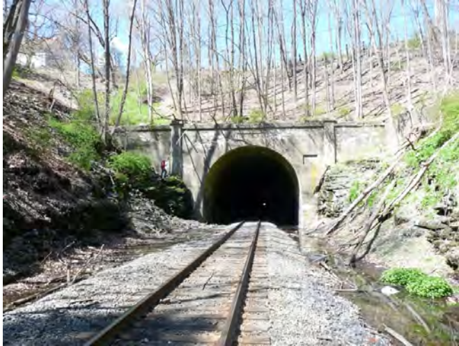
Figure 11. East portal of the Erie Railroad tunnel at Otisville (GPS 41°28'25.1"N/74°32'13.2"W). Intensely deformed Martinsburg shale and sandstone are exposed on both side of the cut
