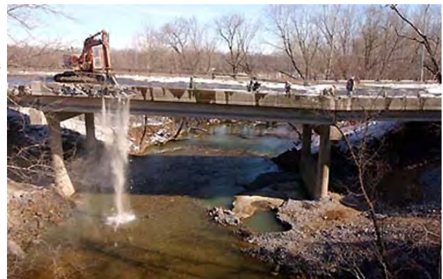
Figure 9. Sinkholes in Bushkill Creek, tilted concrete pier, and sagging roadway of PA 33 in 2001. See Kochanov (p. 139 of this guidebook) for details.
