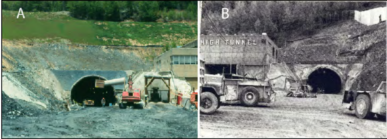
Figure 35. A - South portal of the second Lehigh Tunnel excavated in the Martinsburg Formation, glacial drift, and colluvium. Bedrock dips approximately 40° and is overturned to the southeast; B - North portal excavated in the Bloomsburg Red beds. Bedding is overturned and nearly recumbent. Note the elliptical shape of the tunnel bore, a diagnostic feature of the New Austrian Tunneling Method.
