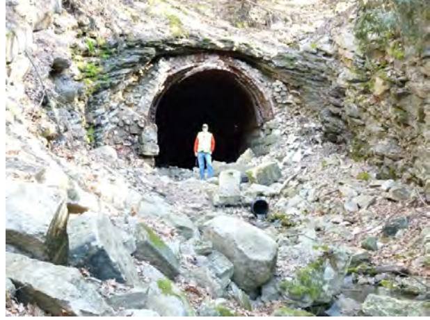
Figure 6. Northwest portal of the abandoned O&W tunnel, about 0.8 mi (1.3 km) east-southeast of Wurtsboro (GPS 41°34'00.0"N/74°28'05.7"W). Bedding in the Shawangunk conglomerate here strikes N33E and dips 26NW. Note the brick lining (with stone facing at entrance) and water flowing from pipe in foreground.
