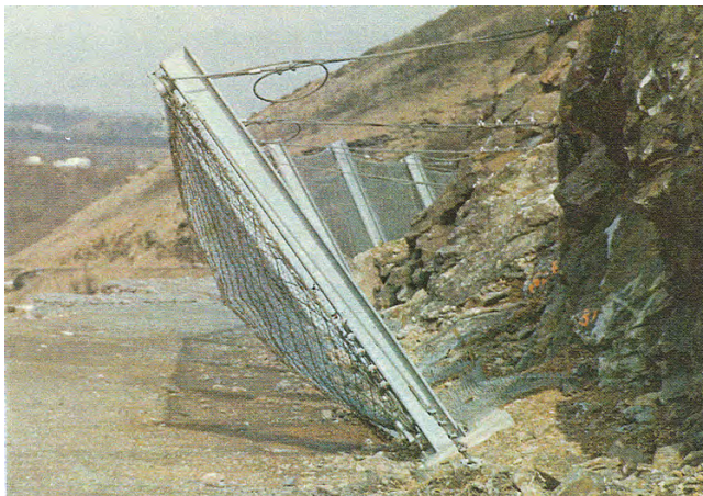
Figure 21. Rock fence installed in the contact area between the Minsi and Weiders Members of the Shawangunk Formation , about 200 ft (61 m) north of the Ordovician-Silurian contact. This is an area of abundant loose talus blocks, possibly within an area of faulting ( Porto and Petrasic, 1996, fig. 23).
