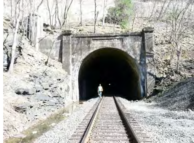
Figure 20. West portal of Erie Railroad tunnel at Otisville (GPS 41°28'41.6"N/74°33'19.9"W). Note outcrop of Shawangunk conglomerate to left of portal. The inscription reads "19—Otisville—08," the year of completion of the tunnel.
