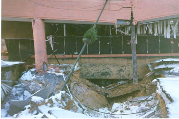
Figure 32. View looking west into sinkhole prior to grouting. Note building support columns suspended in mid-air. The volume of material associated with the column which was lost into the sinkhole can be estimated by comparing with the adjacent column. The slabs below the building are the basement floor. Note the small central bed-rock ridge in the lower left of the photograph.
