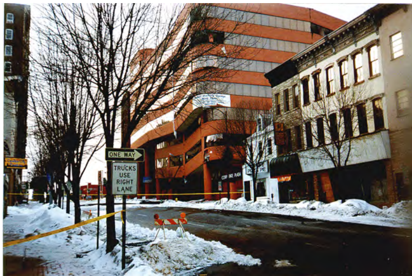
Figure 27. View of Corporate Plaza building looking south on 7 th Street toward Hamilton Circle. Note missing brick support column and sagging facade of building. Also, in upper right, note that the northwest corner of the building has subsided.
