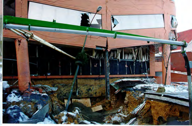
Figure 33. View looking west into the sinkhole at the time of grouting. View shows vertical northern sidewall and underground utilities severed during the collapse.
