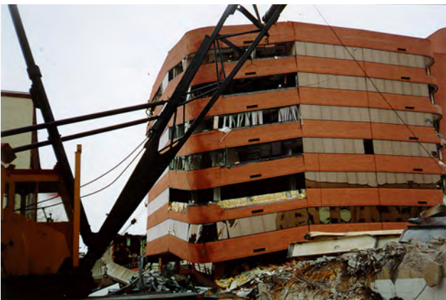
Figure 34. View looking east at the northwest corner of building where support column subsided 1.7 m. Photograph was taken after demolition of the adjacent parking garage.
