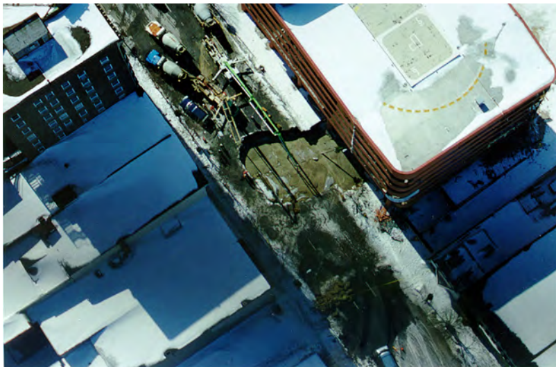
Figure 29. Aerial view looking into the 7 th Street sinkhole during grouting. The sinkhole extends beyond the NW corner of the building at the far right, and below grade to the left under the two medium-height buildings.
