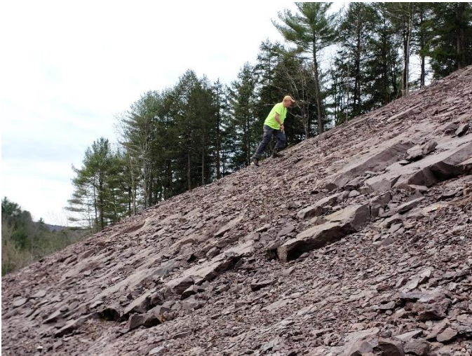
Figure 5.3. Roadcut of Catskill Formation along PA Route 87. Picture is facing west. Catskill sandstone and shale dipping 35°
