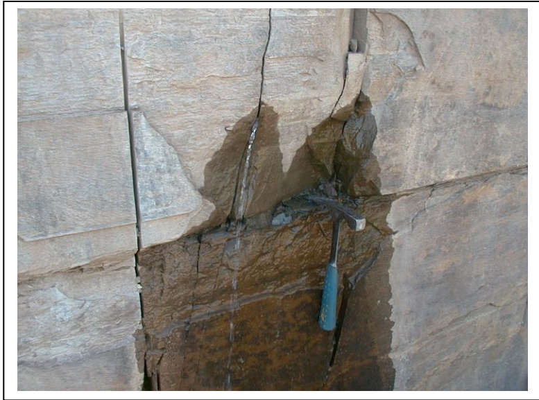
Figure 11A.2. Groundwater discharging from open fractures in a Catskill sandstone. Photo from Kochanov station ff-54, Franklin Forks 7.5-minute quadrangle, Susquehanna County.
